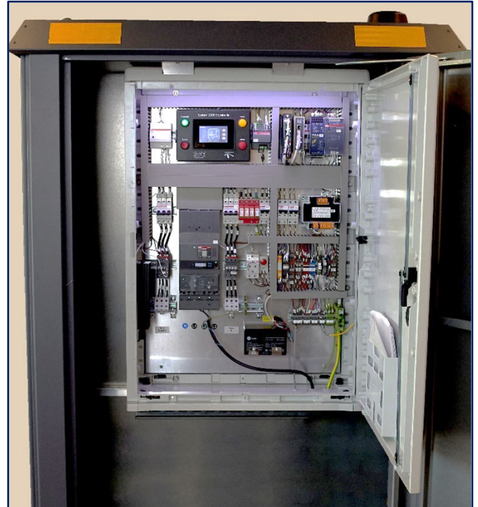
MS-2 in a plastic cabinet mounted in a painted steel outdoor cabinet
