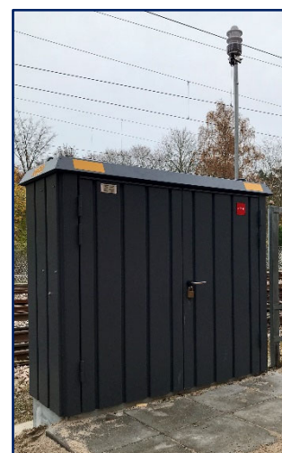
Painted steel cabinet
