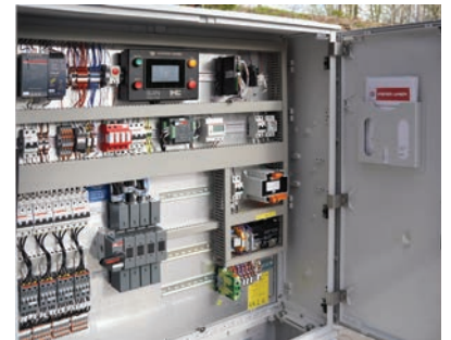
Control cubicle with user interface.
